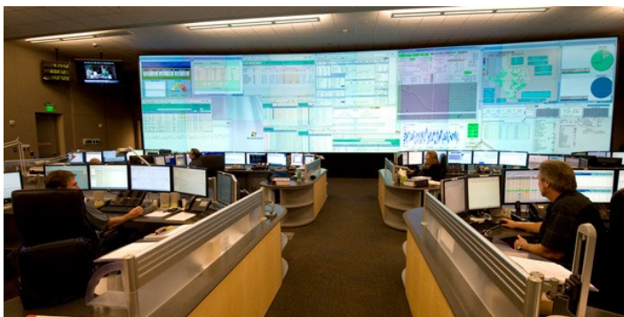
ERCOT control room | ERCOT
